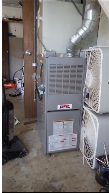
6.0 Item 1(Picture) Air Handler
