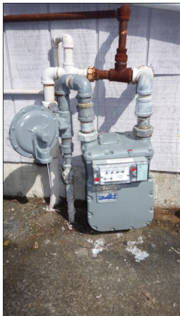
5.4 Item 1(Picture) Gas Meter
