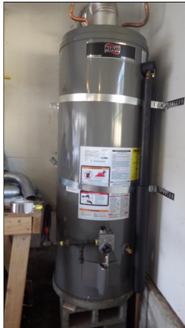
5.3 Item 1(Picture) Water heater
