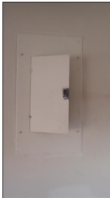
4.0 Item 2(Picture) Electrical panel
