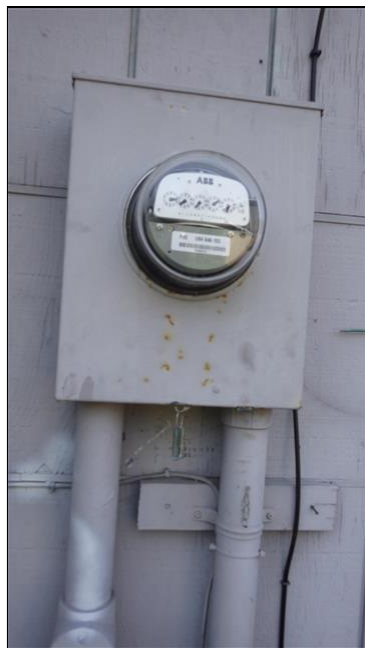
4.0 Item 1(Picture) Electrical Meter
